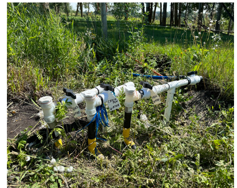
Shallow, buried water infrastructure
